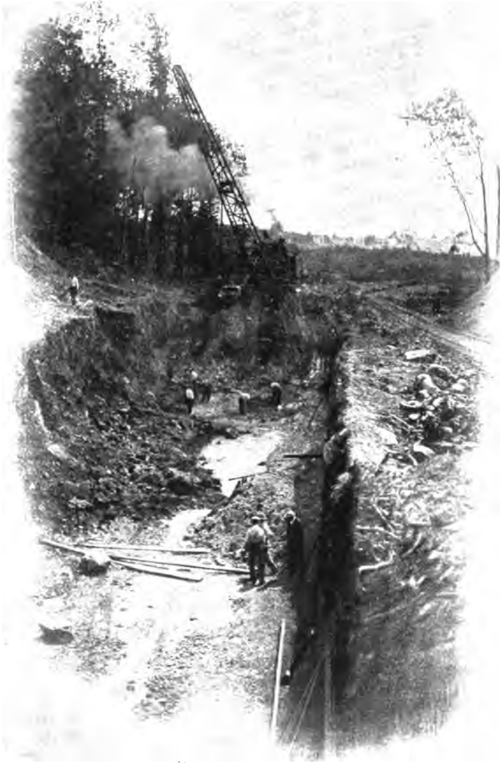
PLATE 186.—Contract 52.—Excavation of Trench for Cut-and-cover Aqueduct with Locomotive Crane and Scraper Bucket.
